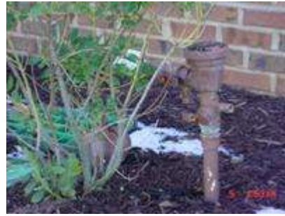
PVB installed too low
