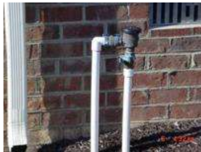
Properly installed PVB Assembly
