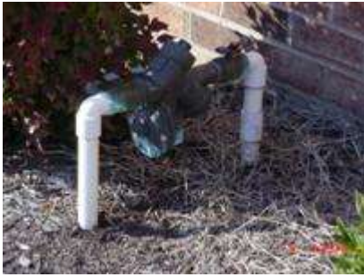
RP installed too close to the ground
