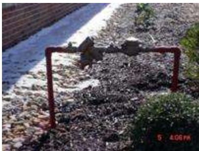
Properly installed RP Assembly
