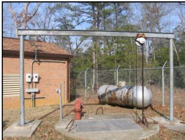
Figure 9 – Norris Pond Sewage Pumping Station
