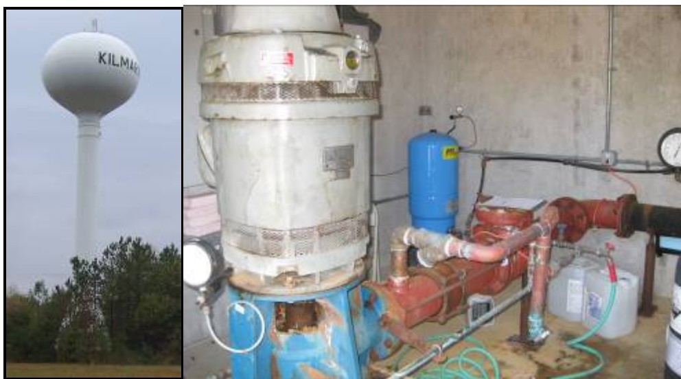
Figure 3 – Radio Well Elevated Tank and Well Pump House Interior
