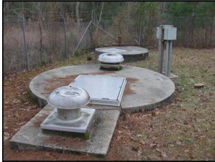
Figure 7 – Wiggins Sewage Pumping Station
