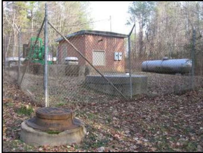
Figure 6 – Harvey Lane Sewage Pumping Station
