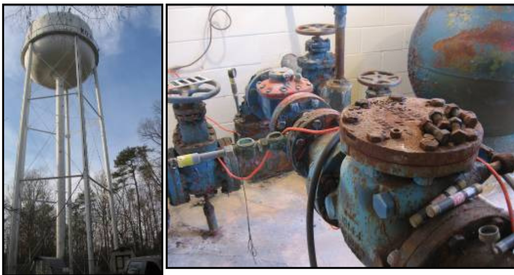
Figure 5 – Hospital Well Elevated Tanks and Well Pump House Interior
